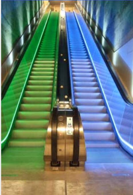
Escalators with LED system at the station "National Theater" in Oslo, Norway
