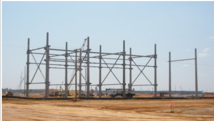
EAF Substation (Alabama Power)
