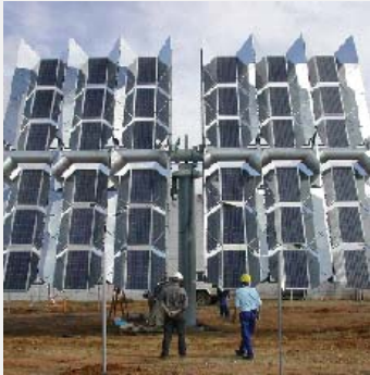
Solar power plants
