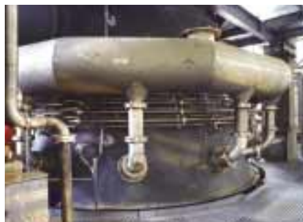
Supplying gasification air to the pre-combustion chamber (Fig. 6)
