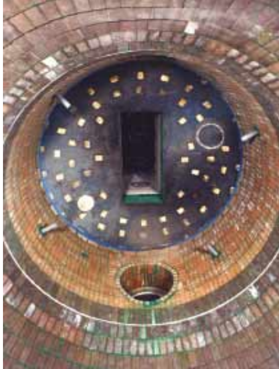
View into a refractory-lined pre-combustion chamber from bottom to top (Fig. 8)
